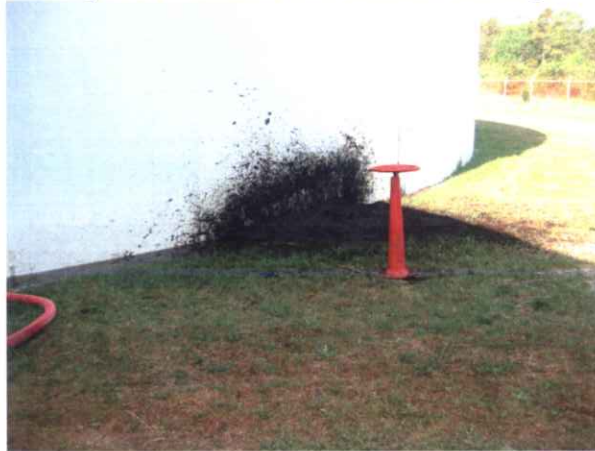
Figure 3-2 - Residual from Clearwell Cleaning
