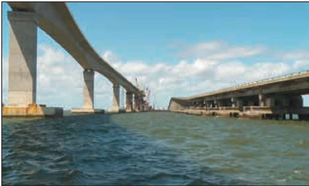
Construction photo of new bridge spanning Oregon Inlet with old bridge alongside the new span.
